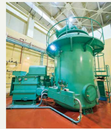
Electron-beam Irradiation Facility (in service)
