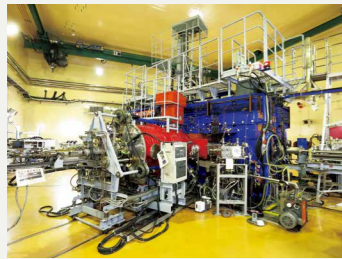
Ion Irradiation Research Facility TIARA (in service)
