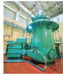
Electron-beam Irradiation Facility (in service)
