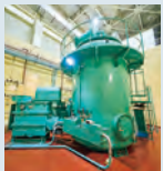
Electron-beam Irradiation Facility (in service)
