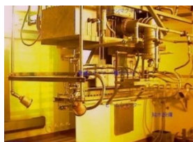
Electron Beam Irradiation Facility
