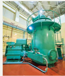
Electron-beam Irradiation Facility (in service)
