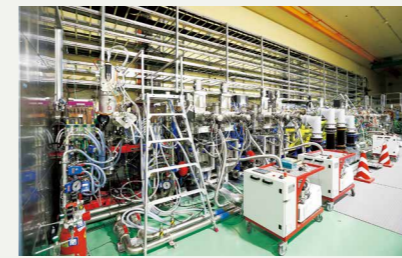
International Fusion Materials Irradiation Facility (IFMIF) Prototype Accelerator (under development)
